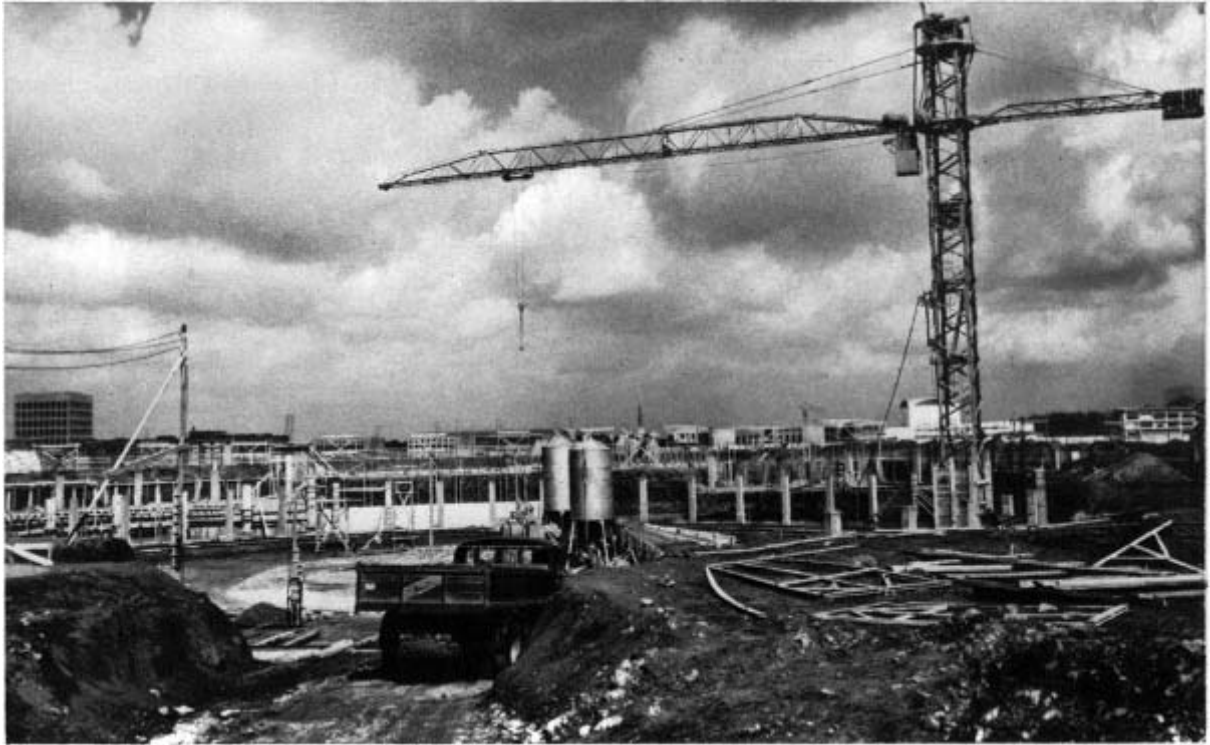
The Palazzo dello Sport under construction. State of work on 15th March 1958.
